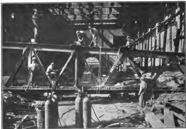
FIG. 77.—Cutting steel with the oxy-acetylene blow-pipe. Portable outfit shown in the foreground.
